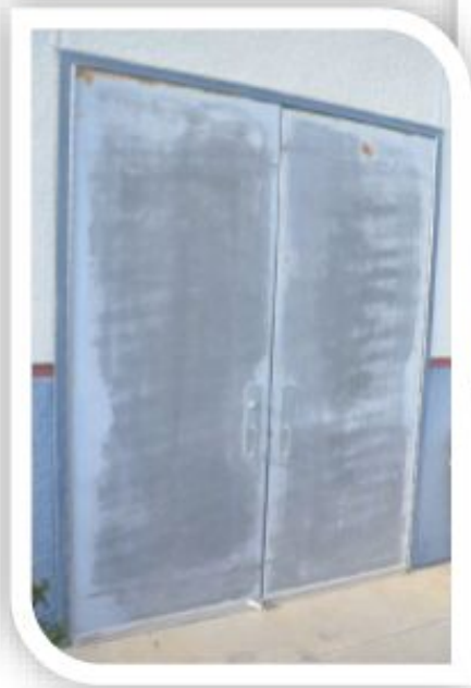
School facilities need repairs
