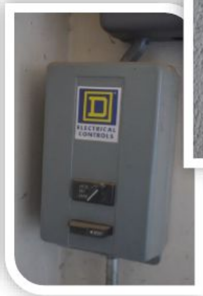
Electrical systems must be upgraded
