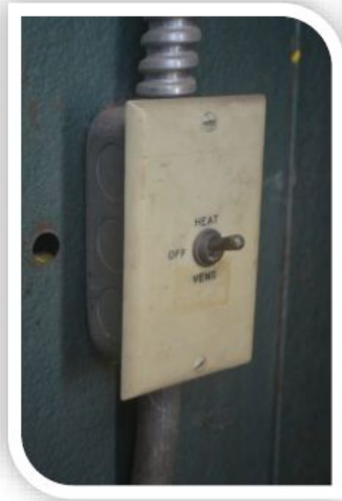
Outdated HVAC systems
