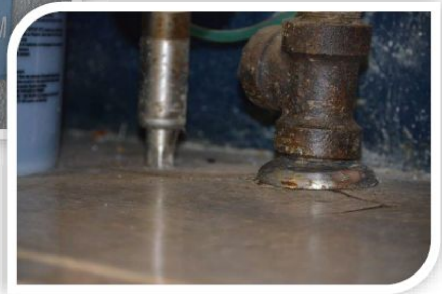
Deteriorating plumbing systems must be replaced
