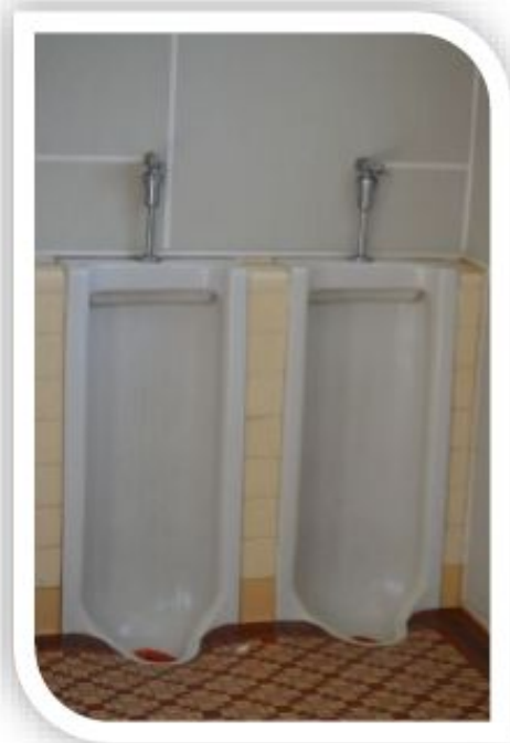
Restrooms need to be modernized
