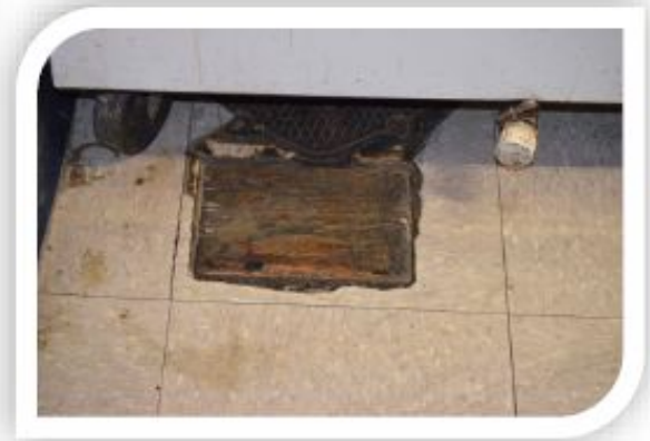
Damaged floors must be replaced
