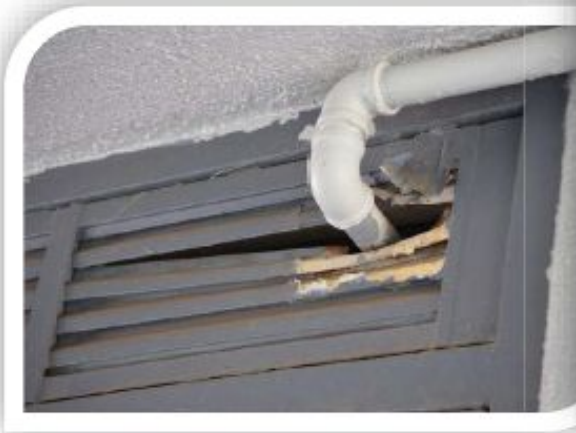
Dry rot buildings need to be renovated
